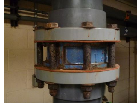
Figure 1.39, Piping bolt corrosion
