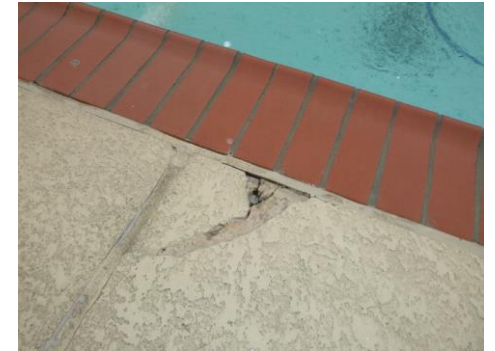
Figure 1.16, Pool deck delamination
