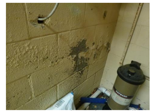
Figure 1.38, Mechanical room wall deterioration
