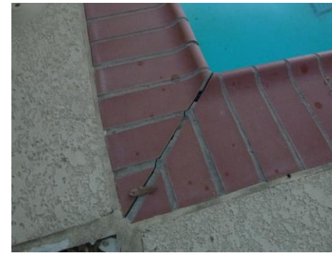
Figure 1.13, Coping stone cracking
