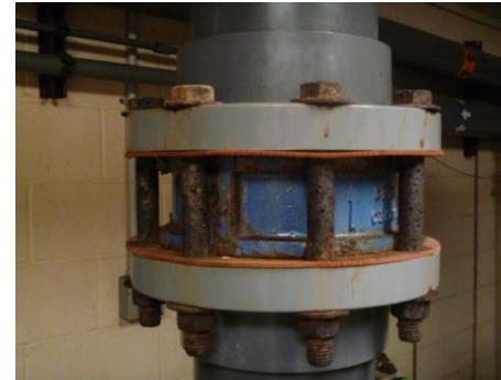
Figure 1.33, Piping bolt corrosion
