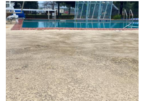
Figure 1.12, Uneven/shifting concrete deck and pool
