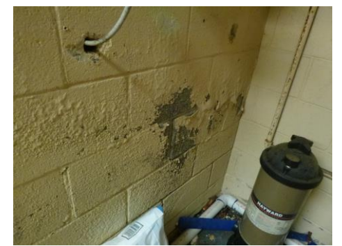
Figure 1.32, Mechanical room wall deterioration
