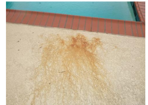
Figure 1.18, Pool deck corrosion
