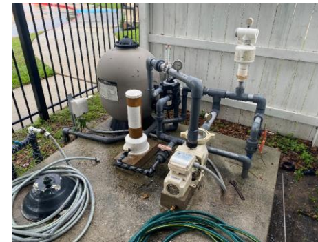
Children's pool mechanical system
