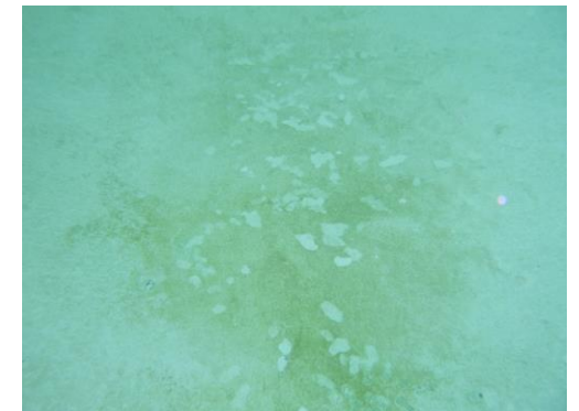
Figure 1.4, Plaster surface etching/delamination
