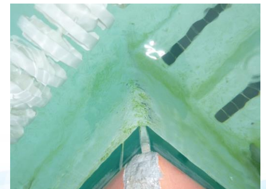
Figure 1.6, Cracking, delamination on corner
