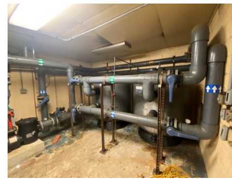
Figure 1.37, Pool mechanical system
