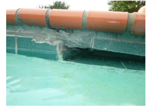
Figure 1.10, Cracked, shifting skimmer basket
