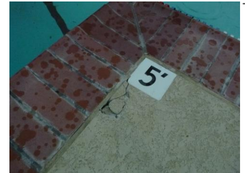
Figure 1.14, Pool deck delamination
