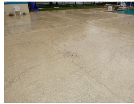
Figure 1.19, Pool deck cracking
