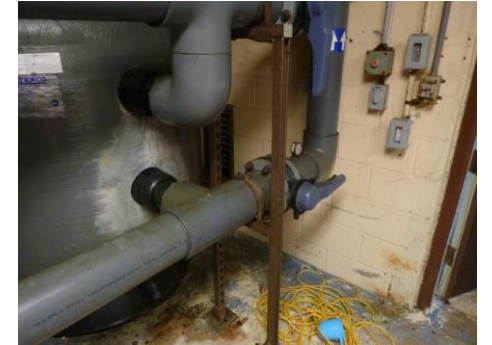
Figure 1.40, Piping support corrosion | area of filter leak
