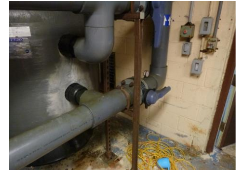
Figure 1.40, Piping support corrosion | area of filter leak
