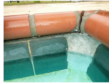
Figure 1.7, Coping stone loose and cracking
