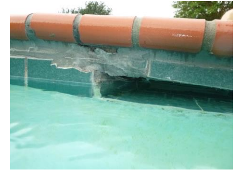
Figure 1.10, Cracked, shifting skimmer basket
