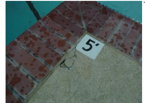
Figure 1.14, Pool deck delamination
