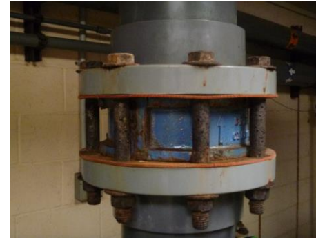
Figure 1.39, Piping bolt corrosion
