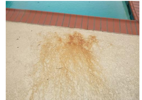
Figure 1.18, Pool deck corrosion
