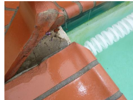
Figure 1.11, Loose/unsecured coping stone
