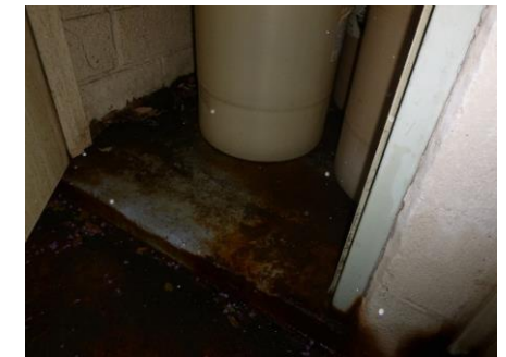
Figure 1.24, Chemical storage room
