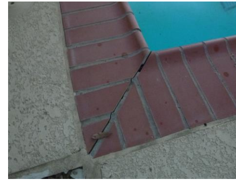
Figure 1.13, Coping stone cracking
