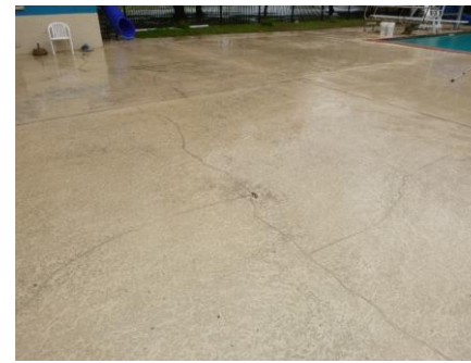
Figure 1.19, Pool deck cracking
