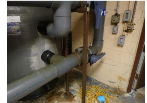
Figure 1.28, Piping support corrosion | area of filter leak
